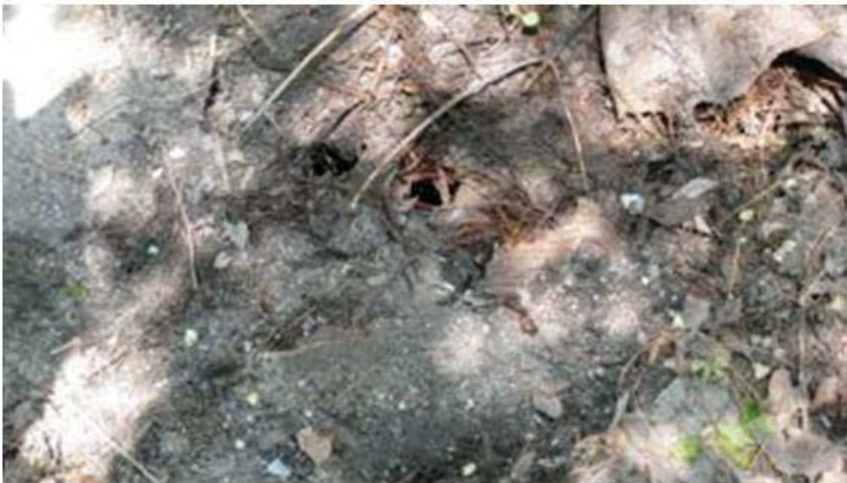
Clogged drain Route 140
