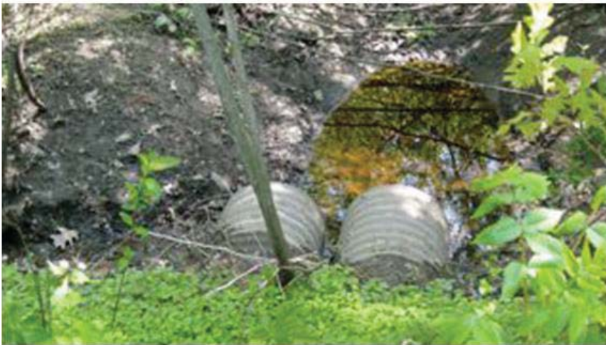
Silted up concrete pipes
