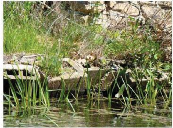
Close up of failed retaining wall
