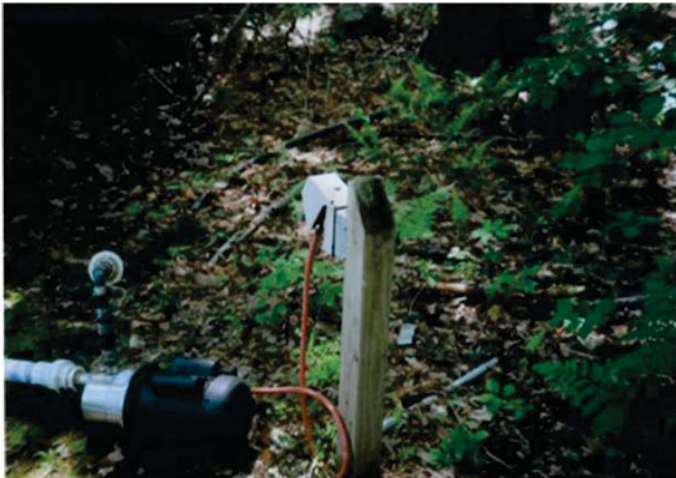
One of several pumping stations found along this stretch
