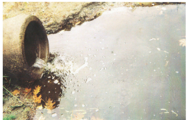
From LakeNipmuc.com website showing one of the offending storm drains.
